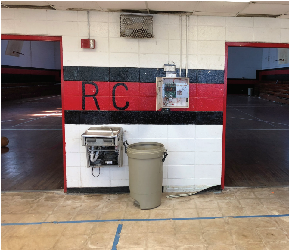
This photo shows the open electrical box at the voting precinct, Cuthbert Middle School. Also, the open plumbing apparatus of the water fountain and ceiling tiles that are not in place are also visible. The facility has not been utilized as a middle school for a number of years.
